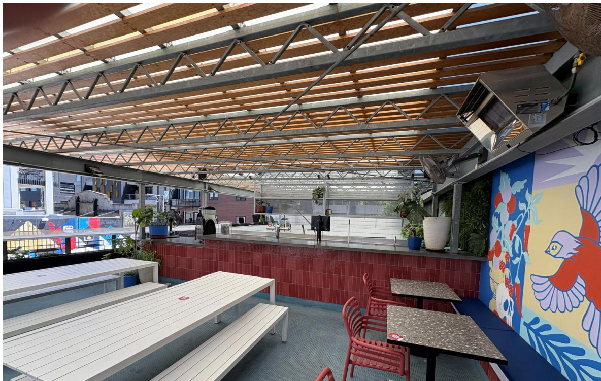
The first-floor bar area. The roofing in this area was very lightweight polycarbonate, with some wooden slats. We do not anticipate notable acoustic attenuation from this system.
