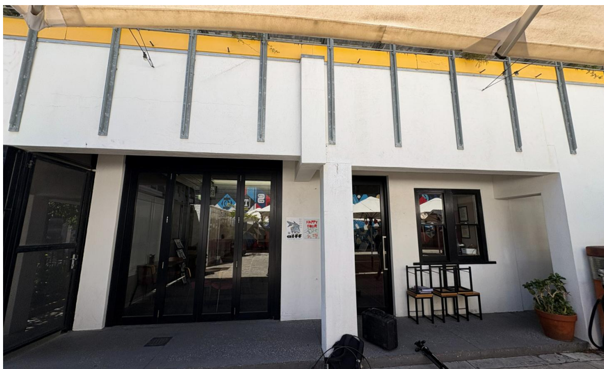
The front entrance of the venue. There are typical walls/doors/glazing systems, however, inside, the ceiling system is virtually open (shown later within this appendix).
