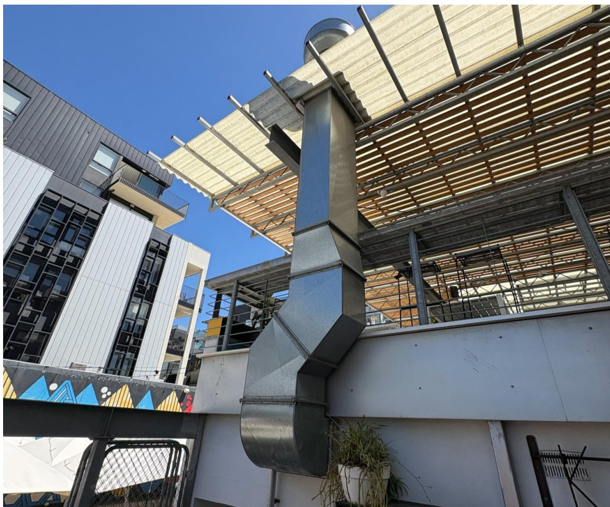
The external extractor vents on the roof area. Currently, this just has an on/off switch, and no speed controller.
