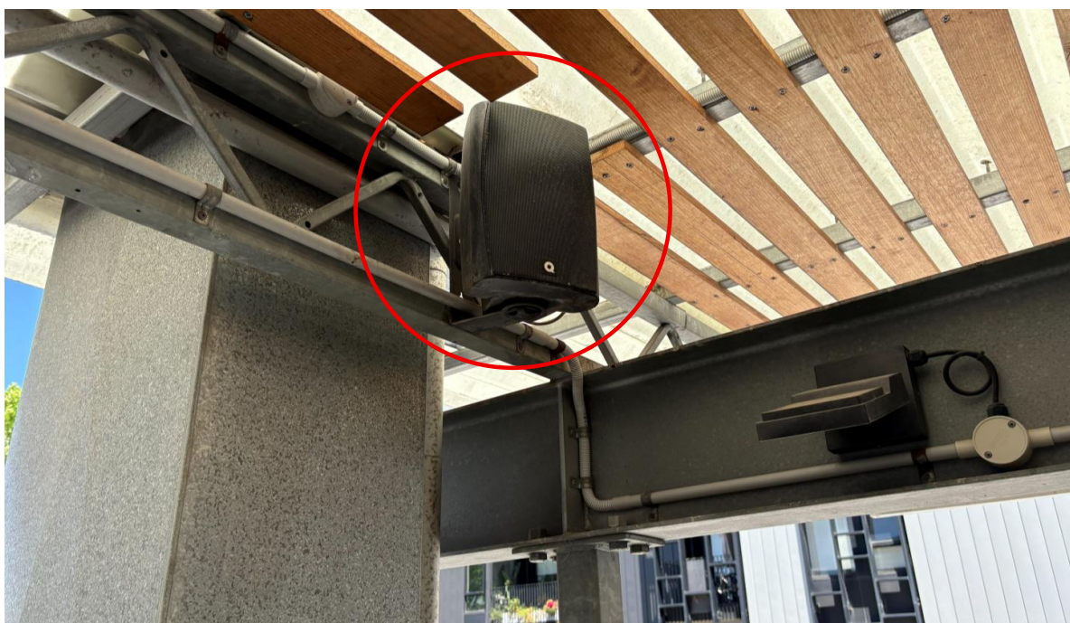
One of the speakers mounted in the first-floor area, behind the bar.
