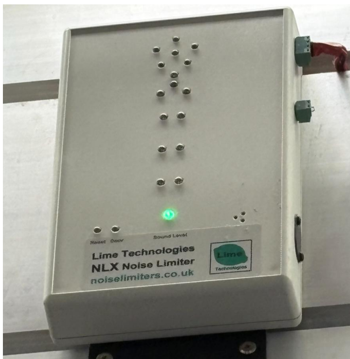
The Lime Technologies NLX noise limiter already installed on site.
