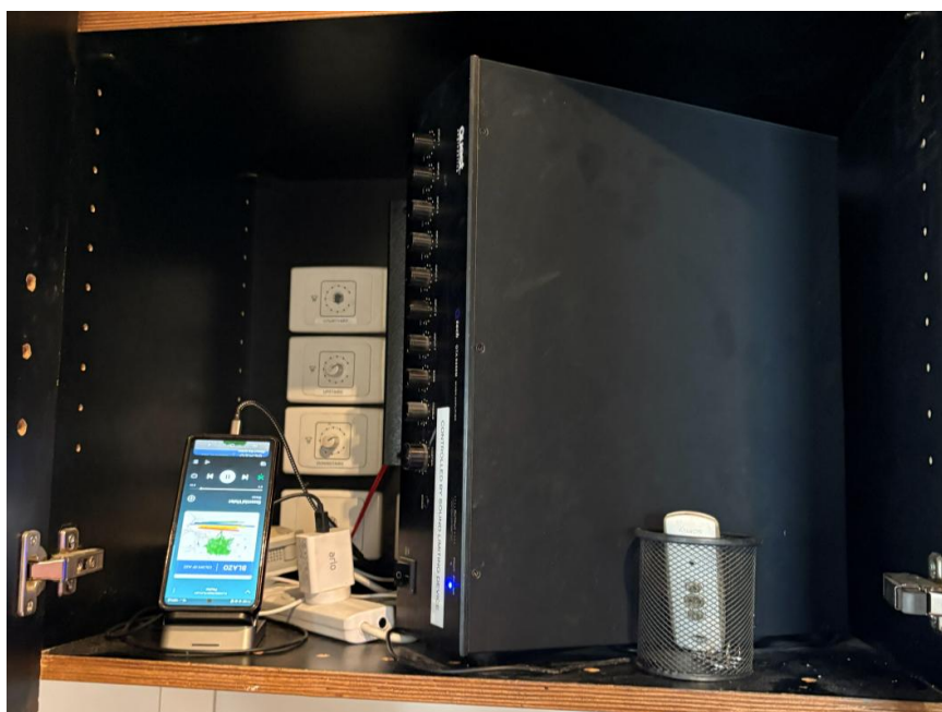
The amplifier system is located within this cabinet. Currently, there are independent controls for the bar above and the café below.
