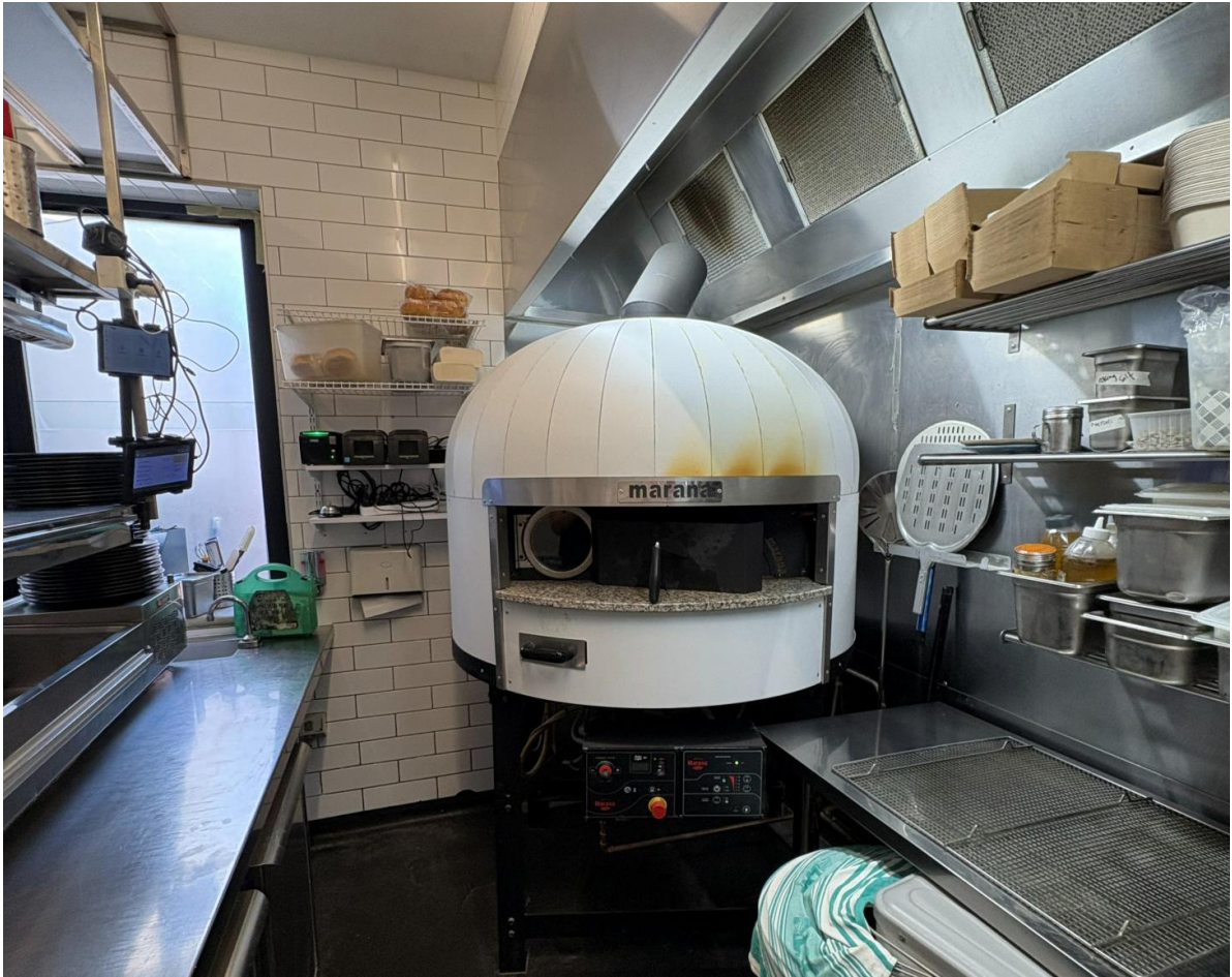
The pizza oven and kitchen extraction system was the main equipment noted during our inspection. This is connected to the external extraction system.
