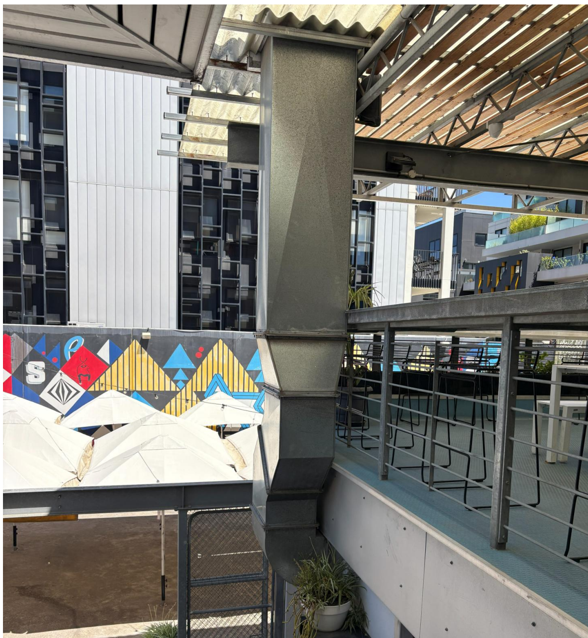
The extractor system used for the pizza oven. This was the only mech identified on site.
