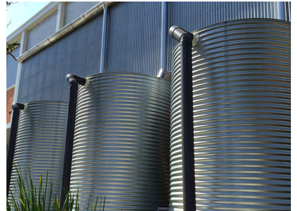
Image - Harvesting roof water for reuse
