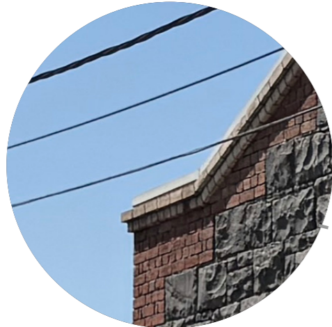
DATUM OF PARAPET CAPPING TO THE HERITAGE INFORMS A STRONG PODIUM AND ARTICULATED DETAIL OF THE FACADE
