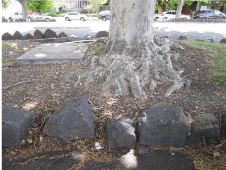
Figure 7: Damage to the median border caused by roots of the London Plane.
