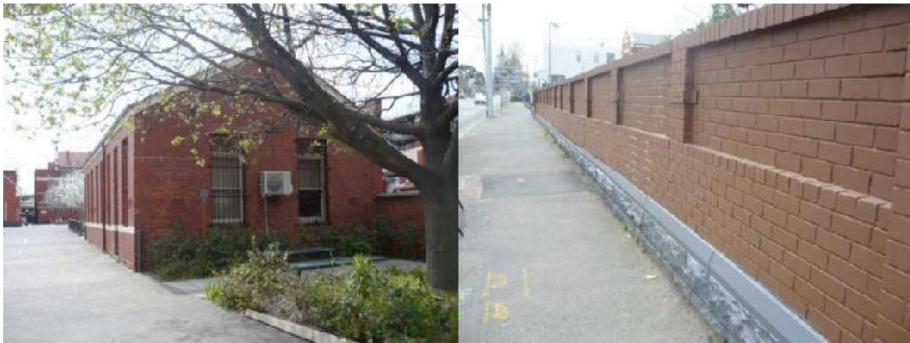
At left, outbuilding at rear of Presbytery. At right, brick fence with original (c. 1911) bluestone base.
