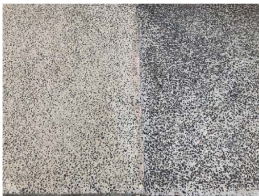
NEWLY LAID PANEL DOES NOT MATCH QUALITY & FINISH OF ADJACENT BAY - NOT ACCEPTED
