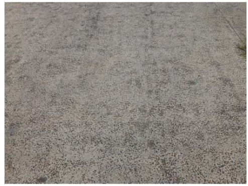
UNEVEN & UNDER EXPOSED - NOT ACCEPTED
