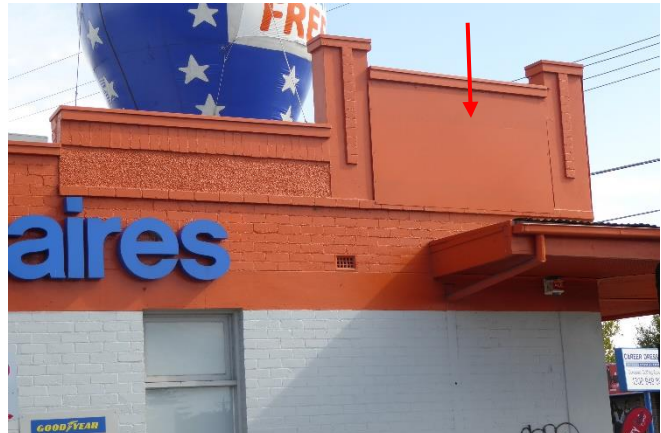
Encourage removal of paint and fixed rendered panels on parapet
