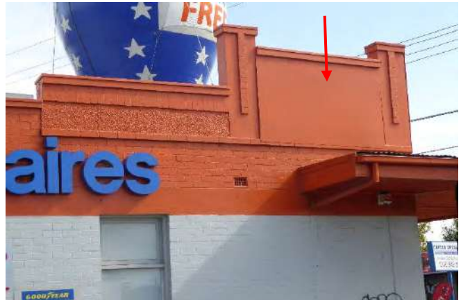
Encourage removal of paint and fixed rendered panels on parapet
