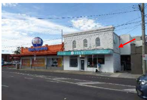
The entire west (side) elevation of the former Butcher Shop (HO71) remains exposed
