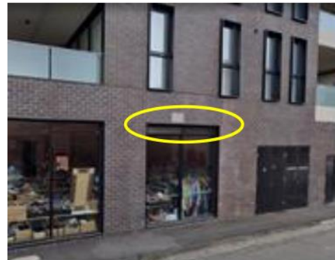
Figure 3: Ventilation louvres – external view
