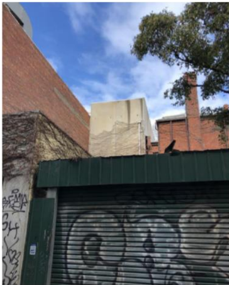
Figure 8 Another view of the north side with (from left to right) brick west wall of 10 Peel Street, concrete slab north wall of 8 Peel Street, and rear brick wing with chimney of 6 Peel Street
