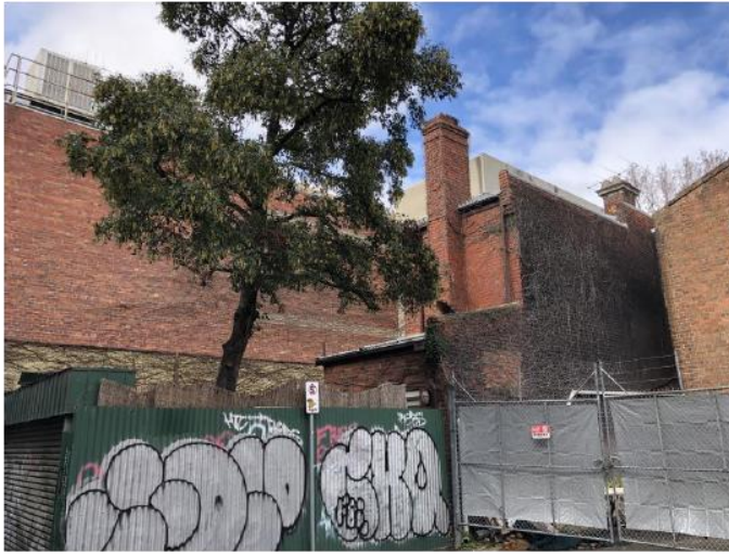
Figure 7 North side of subject property with (from left to right) brick west wall of 10 Peel Street, concrete slab north wall of 8 Peel Street (visible behind chimney), and rear brick wing with chimney of 6 Peel Street
