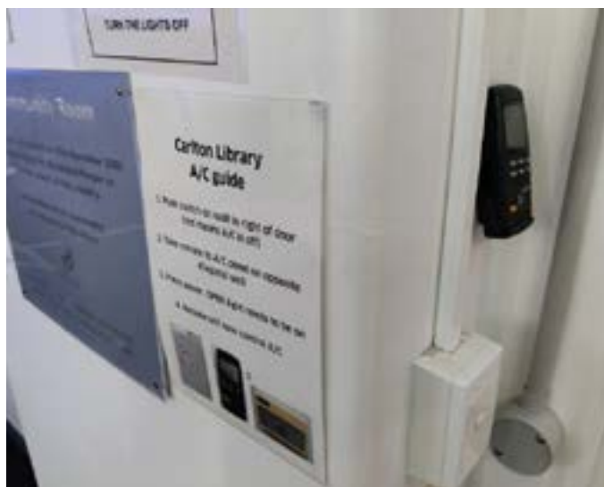
Heating and cooling control
