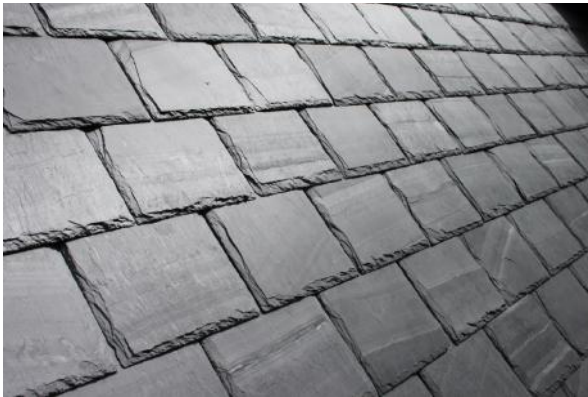
RF1 – Welsh slate roof tiles to match existing. CL – Welsh slate tile wall cladding to match existing roof tiles.
