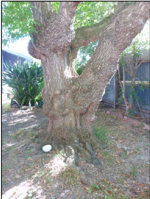
Tree #1's base; some exposed structural roots show early indications of decay.
