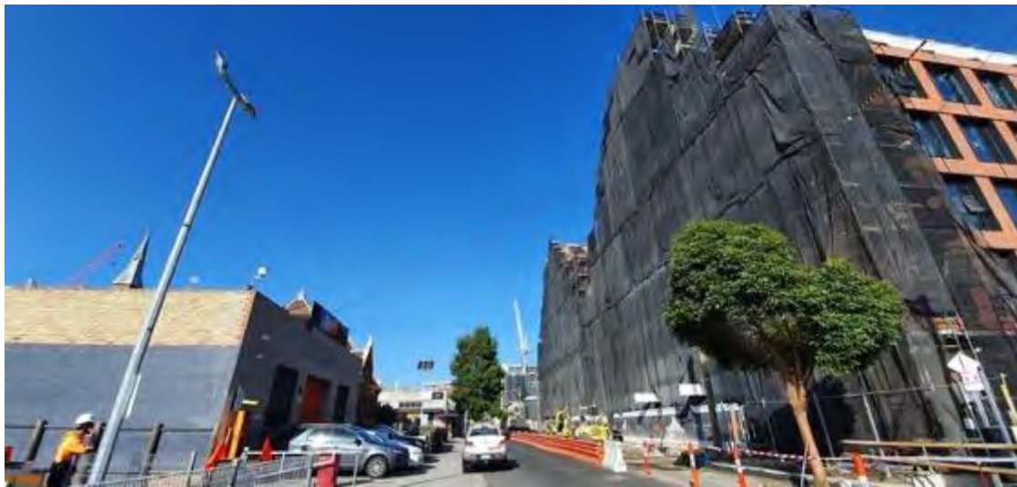
Figure 24. Current development across the road is very dominant, sheer, but references contextual material and roof forms and is separated from the heritage site by the street. Source: Trethowan Architecture.
