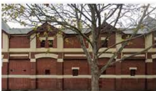
Existing Colour Match - Utilising the existing Ticketing Box for colour matching of façade materials
