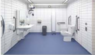
Accessible WCs - The inclusion of Changing Places and Accessible WCs within the facility
