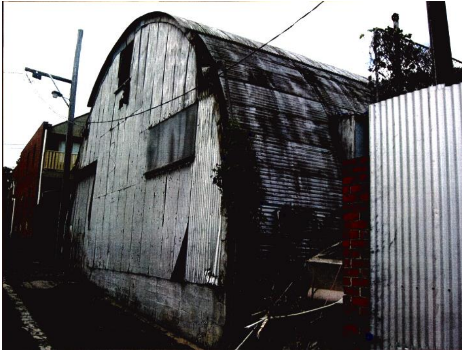
Figure 6. The west and south elevations of the vacant building in April 2006 prior to conversion (YCC BP).
