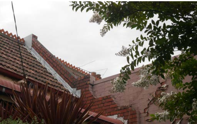
Image 9. View of chimneys above the roofline at the interface between 495 and 497 Swan Street.
