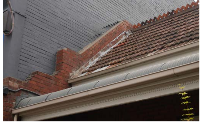
Image 8. View of the roofline at 493 Swan Street as it interfaces with 487-491 Swan Street to the west.
