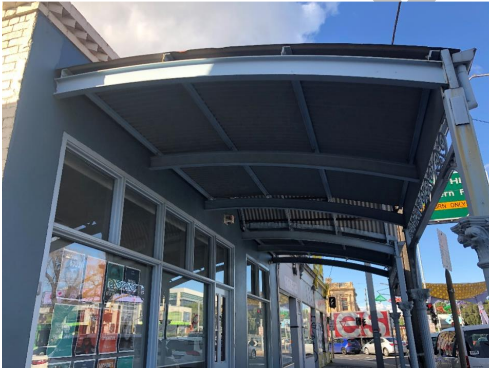
Figure 7. Looking east to the canopy at 211-213, showing later steel structure above cast iron verandah posts.
