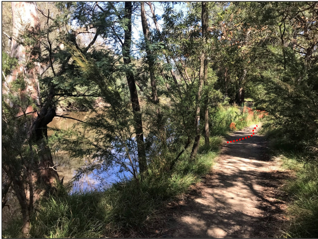
Image 1. Taken from next to Tree 81 (left) looking west. The red dotted line shows the approximate length of the newly appeared soil cracking.
