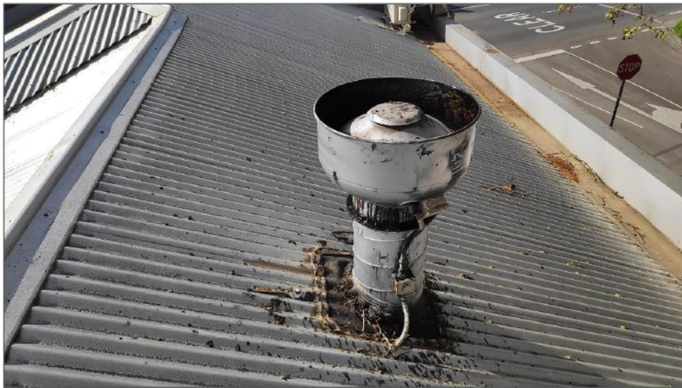
Figure 4 Key Noise-Generating Mechanical Plant Items – Kitchen Exhaust Fan
