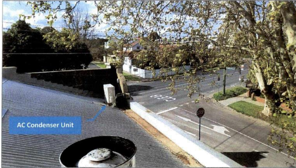
Figure 5 Key Noise-Generating Mechanical Plant Items – AC Condenser Unit
