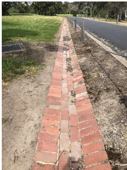
2019, S facing image showing a spoon drain comprised of potential re-used bricks.
