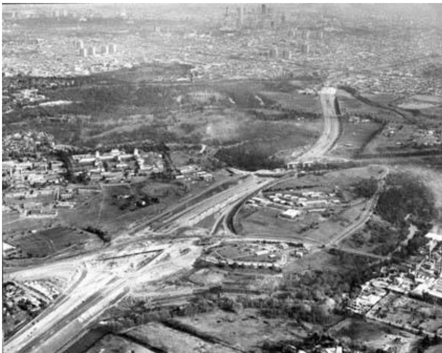
c. 1972, The Eastern Freeway - Stage One under construction, looking towards the city. The Chandler Highway alignment is in the foreground with Willsmere to the left.
