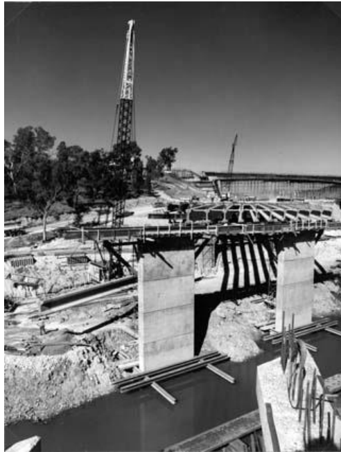
n.d., The Yarra Boulevard Road bridge under construction, with the pylon of the Yarra River bridges in the foreground. Source: National Archives of Australia.
