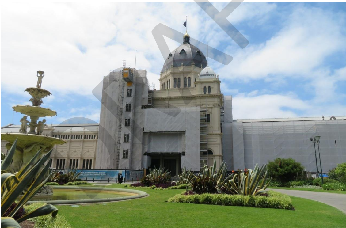
Figure 7 South façade of the REB c. 2019 during the 'Protection and Promotion' project
