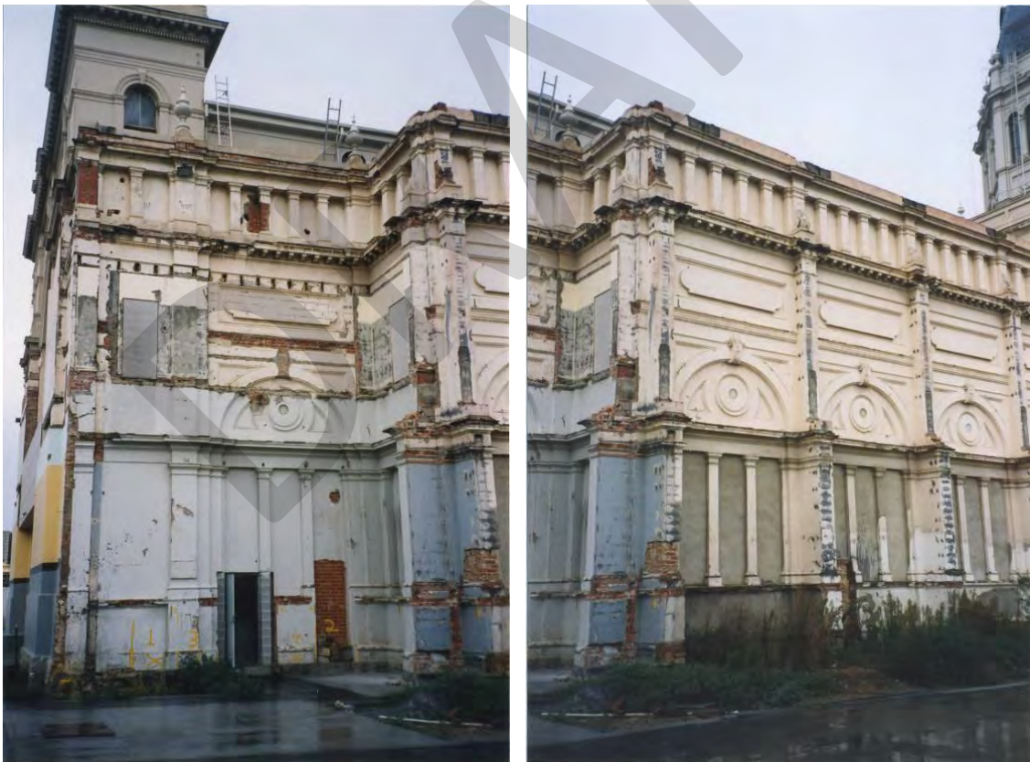
Figure 39 Late 1990s images of the western elevation of the north transept, showing condition after removal of annexe
