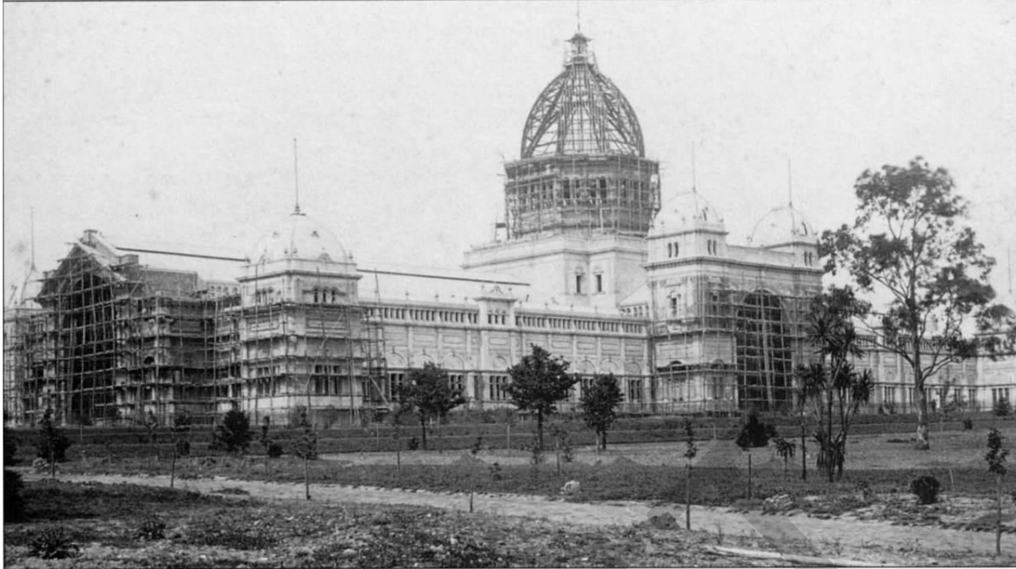
Figure 20 The Exhibition Building under construction c.1879. The southern section of the Carlton Gardens was in the course of being laid out by William Sangster contracted to execute Reed's design. As the ground sloped markedly from east to west, a large terrace was constructed in front of the Exhibition Building to provide a platform for the promenade and flower beds, although the present form suggests that this was incompletely executed Source: Reproduced from Civilising the City: A History of Melbourne's Public Gardens
