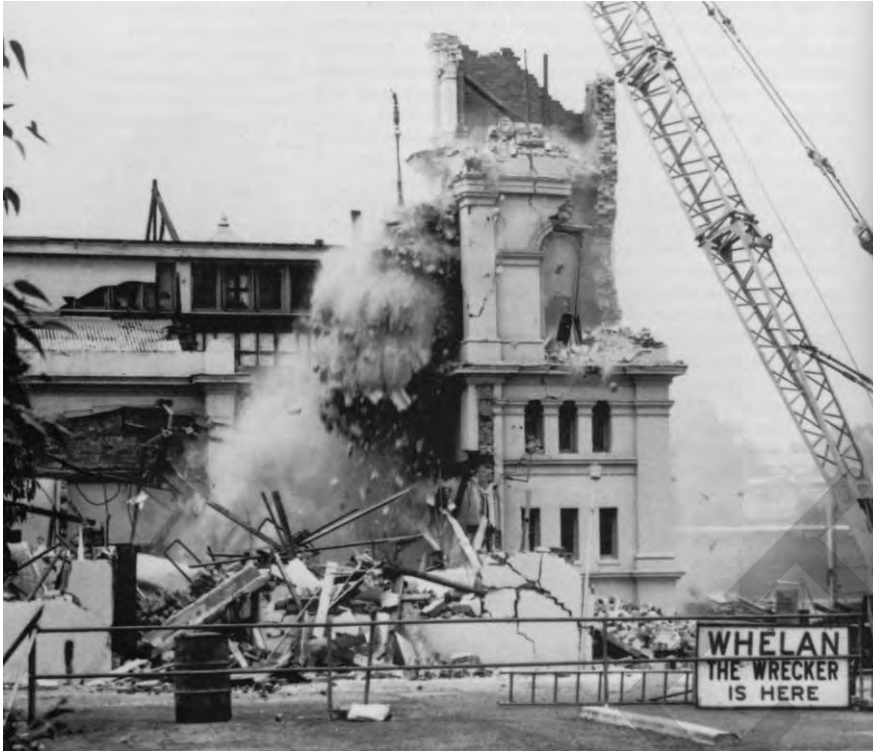
Figure 98 Demolition of the Royale Ballroom in the Eastern Annex of the Exhibition Building, 1979 Source: Reproduced from Victorian Icon, The Royal Exhibition Building Melbourne
