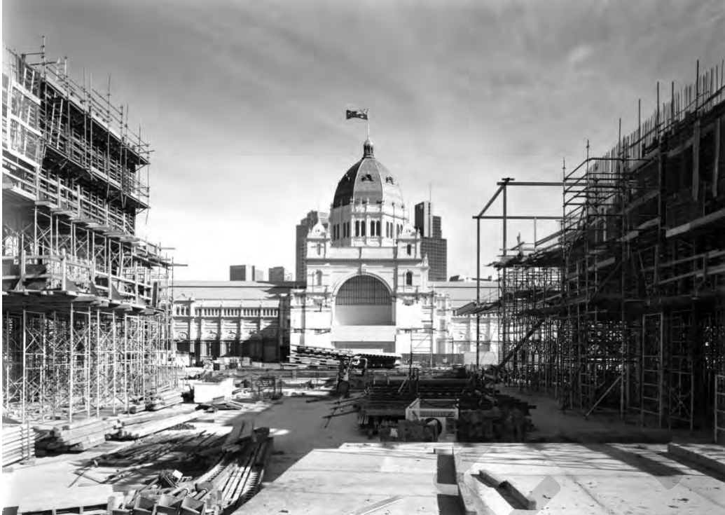
Figure 40 View of north elevation of Royal Exhibition Building during construction of Melbourne Museum, 1998 Source: H2000.60/1, Ian Hill, State Library of Victoria
