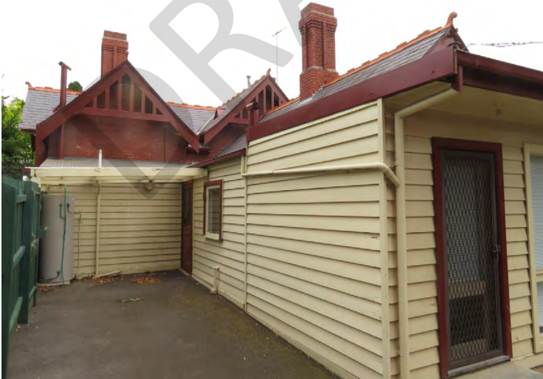
Figure 81 View of the south-east section of the Curator's Lodge, with the former bath house, infilled verandah, rear skillion addition (right) and modern pergola
