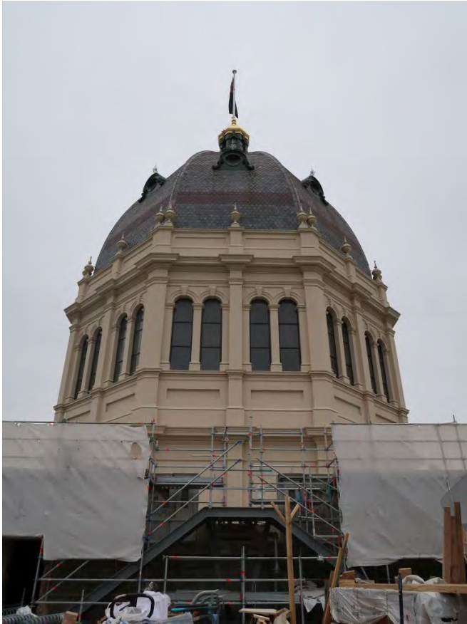
Figure 15 The dome and cupola viewed from the south at promenade level; note the dome and cupola repair works are complete and works for construction of the promenade deck are underway
