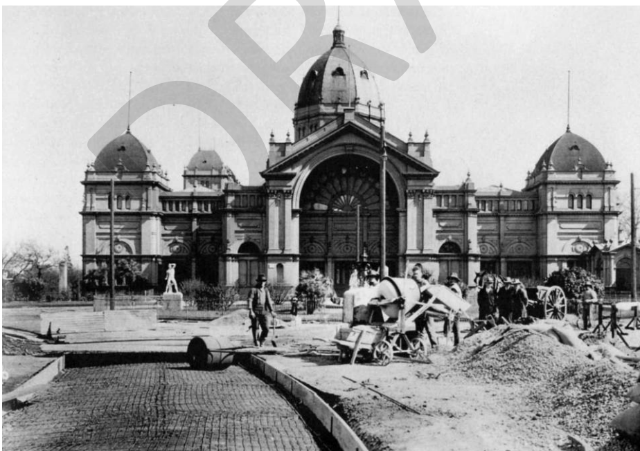
Figure 83 Pouring concrete for the Nicholson Street entrance driveway at the Exhibition Building in the 1920s. Note that the French Fountain and statuary dating from the Great Exhibitions are still clearly visible. Source: Reproduced from Victorian Icon: The Royal Exhibition Building Melbourne
