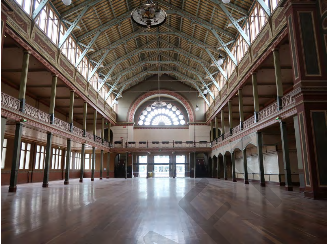
Figure 23 View of the interior of the north transept; the kiosk is at right
