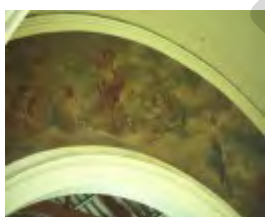
royal exhibition buildings nicholson street carlton detail of wall painting
