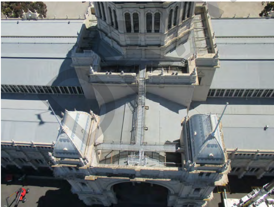
Figure 14 View of the dome base above the southern entry c. 2015, prior to the installation of the promenade deck
