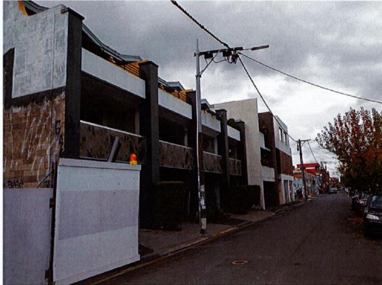
Figure 9 No. 63-69 Rose Street, 3 storey town houses. Note the site under construction on the left – I am not aware of what is being constructed.
