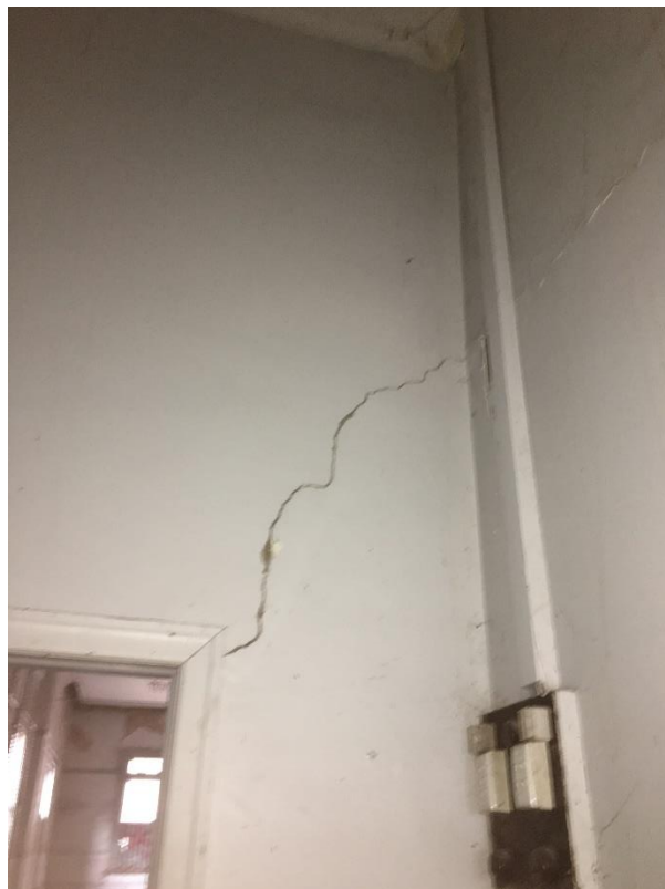
Photo 17: Other side of wall shown in photo 16, crack is on both faces of internal brick work wall.
