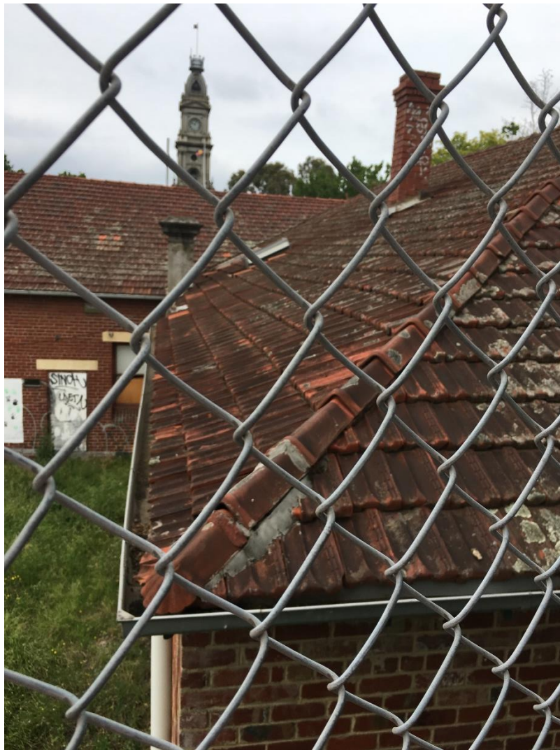
Photo 5: Tiled roof at North-East corner. Tiles to be removed, repaired and re-pointed. Eaves, gutters and downpipes to be replaced.
