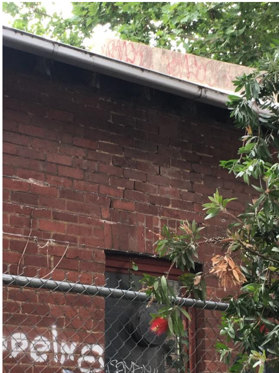
Photo 7: North wall has new formation of cracking above lintel, cracks are new and was not observed and documented in previous report.
