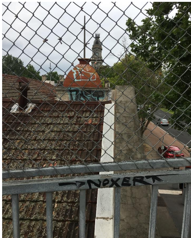
Photo 2: Turret structure above main entry. North and South gable walls warped and leaning outwards. By observation current state looks similar to previous report photos.
