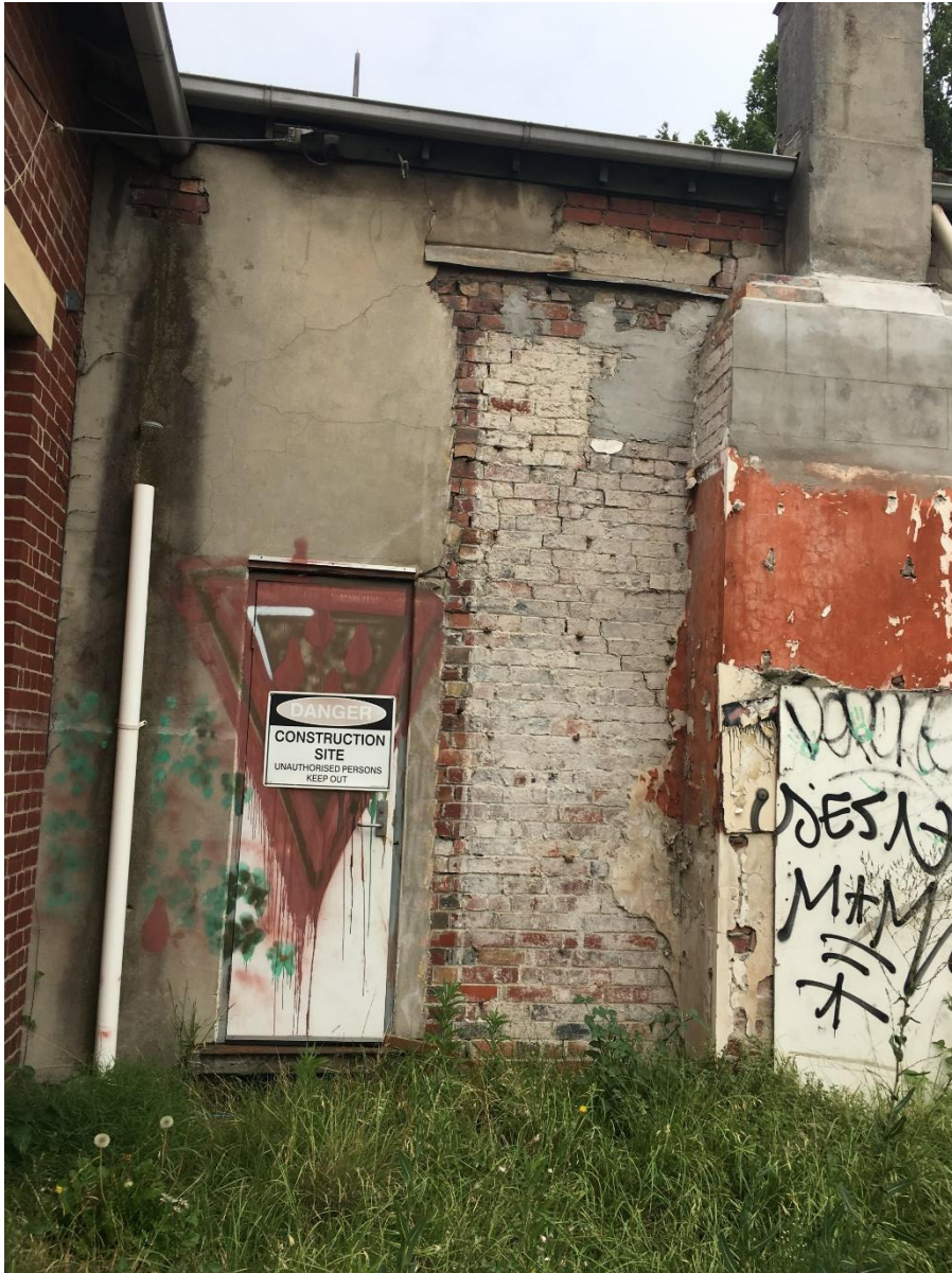
Photo 15: Rear Exit at east end of main entry hall. Disconnected downpipe and heavy water damage to external render. Single story toilet block has been demolished and external brickwork exposed which is heavily cracked.
