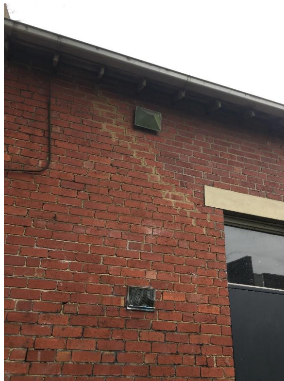
Photo 10: South-West corner of Hall. Foundation may have dropped. Wall repaired previously, in buildings current observation repair is starting to crack again at top of brick wall.
