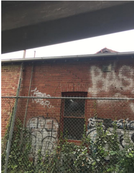
Photo 6: North Wall looking externally. Re-constructed where ivy had penetrated brick courses, Large crack right through lintel & reflective cracks right along north wall.
