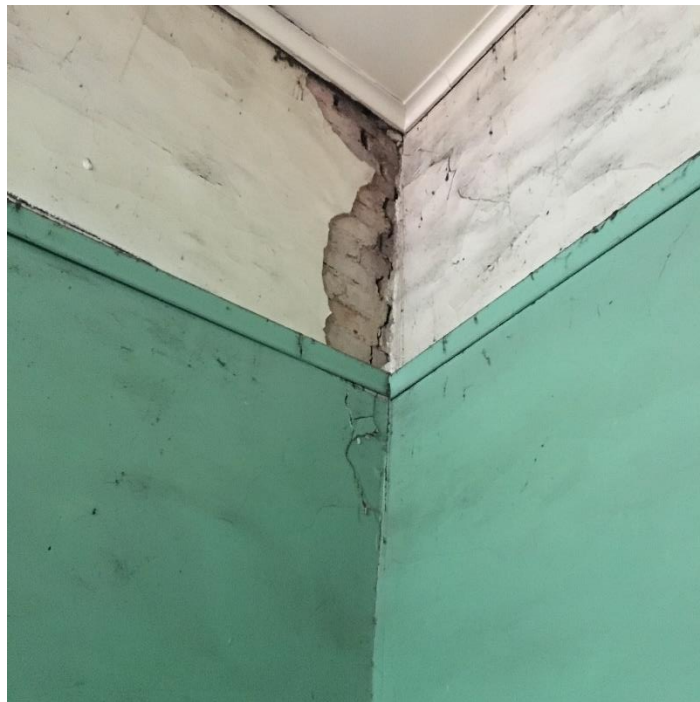
Photo 22: Large cracking in room 4 where brick wall meets each other at corner. Was not overserved and documented in previous report.
