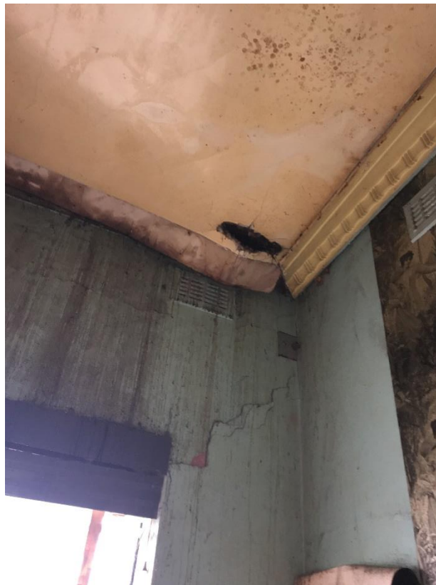
Photo 24: Room 12, first floor at corner of south east wall, cracks starting to form, and roof is starting to fall down from heavy water damage. Walls are heavily water damaged also with large amounts of rot.
