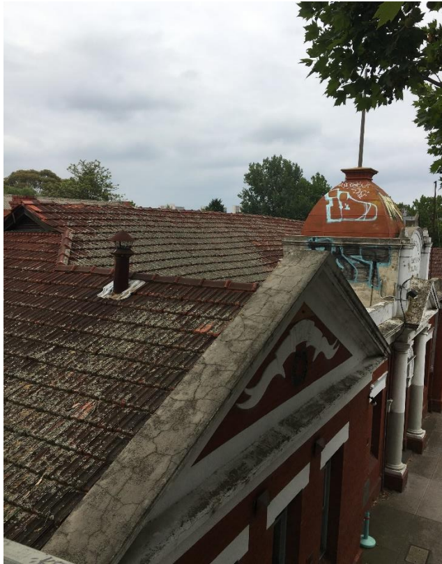
Photo 3: Main roof viewed from North-West. Remove tiles, re-level battens and re-instate tiles, central part of roof looks bowed which was also stated in previous report.
