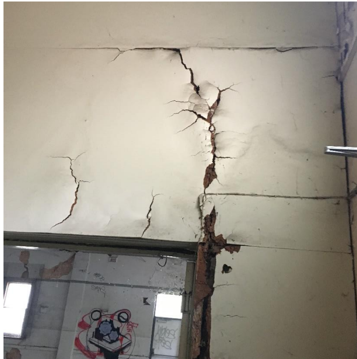
Photo 23: Large cracks & rotting of timber walls from settlement movement and water damage. Crack was observed at entrance of room 8 & 6.
