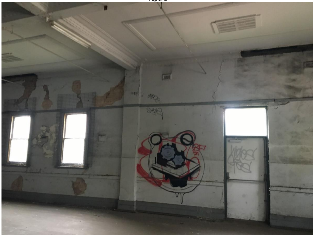
Photo 13: Looking at South Wall internally, cracks have not been repaired internally and run continuously across whole wall. Also brick ties can be seen just below roof level. Patchwork was only done externally, and no work has been done on internal face.
