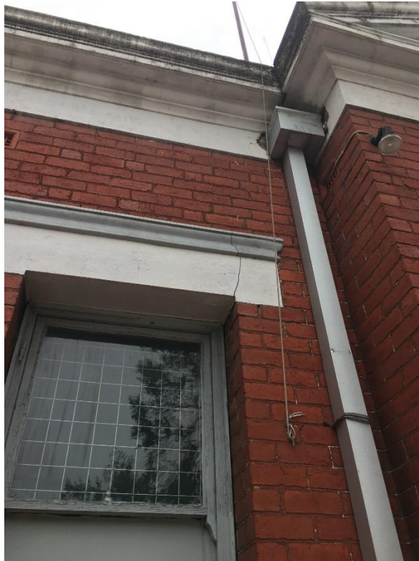
Photo 21: Front Façade West Wall (Hoddle St) has a large crack through lintel at support where lintel is bearing on brickwork. Was not observed and documented in previous report.
