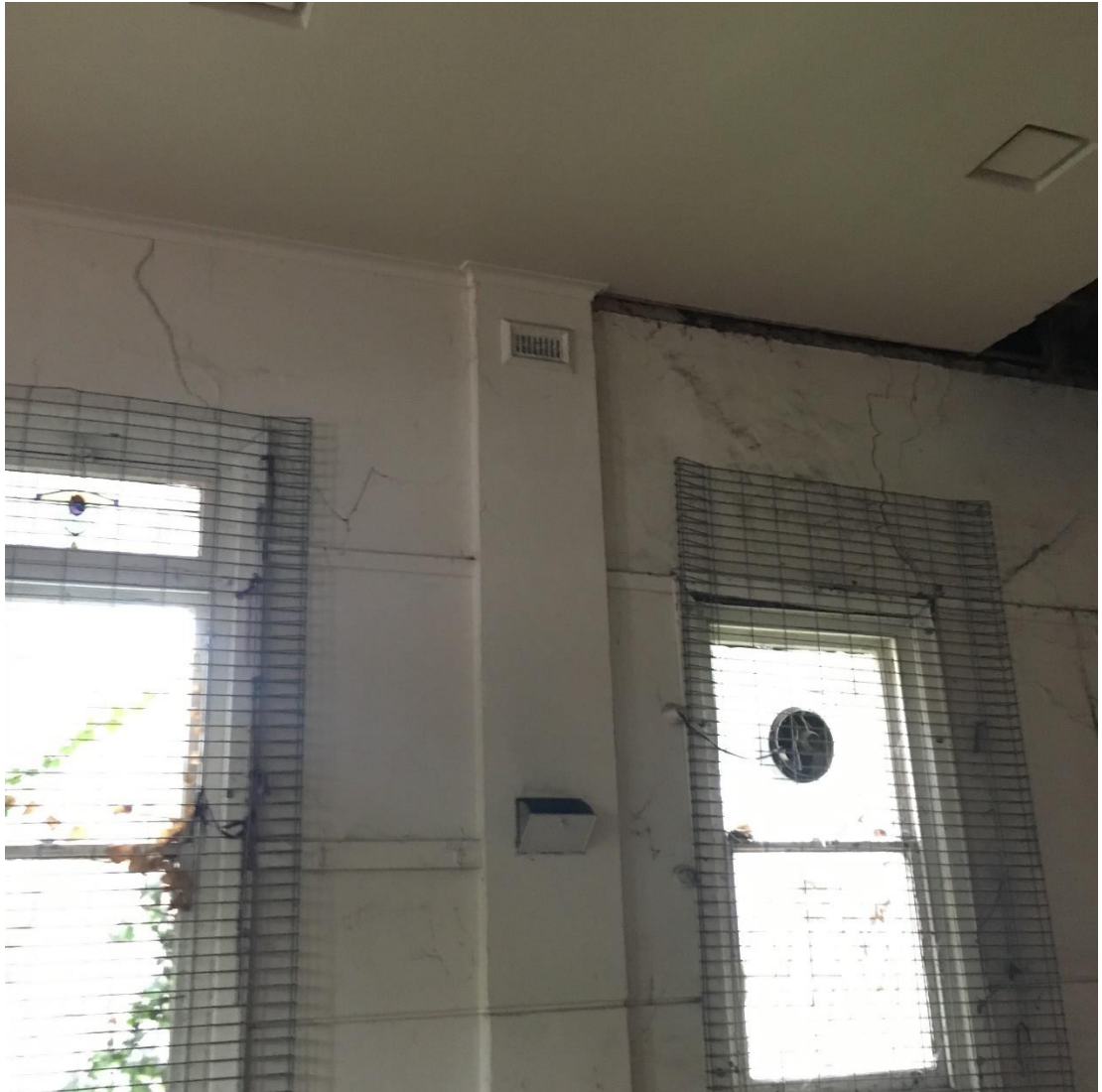
Photo 8: North Wall looking internally both previous photos 6 & 7 are the same cracks viewed externally.
