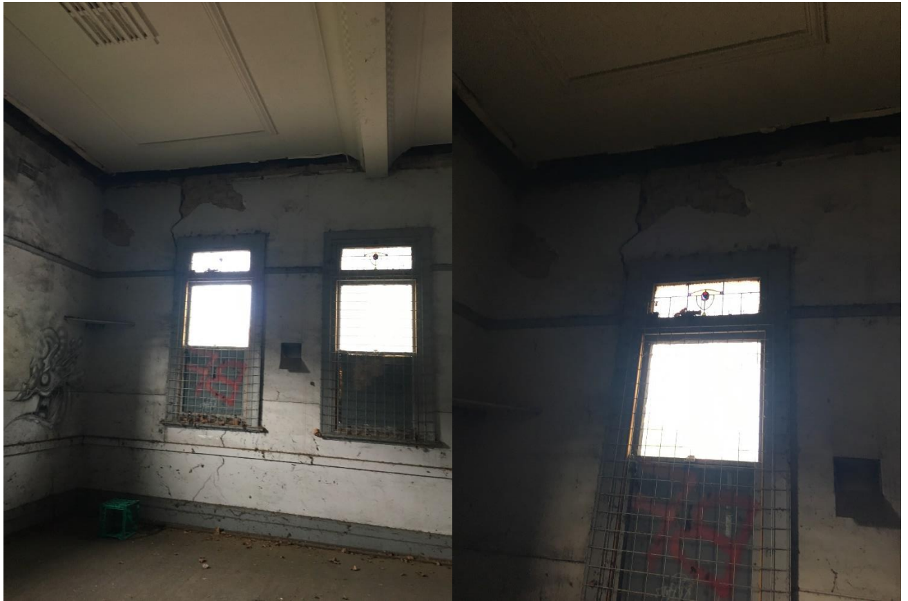
Photo 12: South-West corner of Room 9 (Hall). Crack to west wall not repaired, internally. Crack looks to have got larger compared to the photos in previous report.
