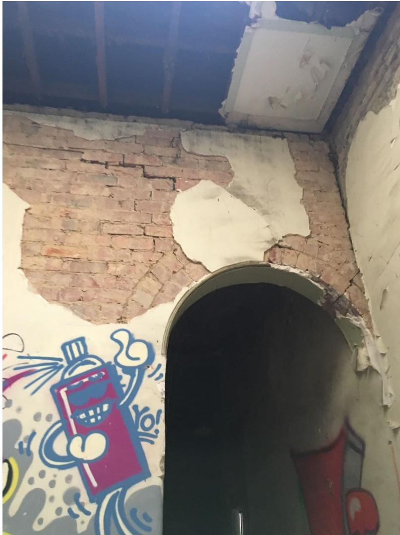
Photo 20: Internal arch leading from room 8 to 7, crack looks to have got worse since previous report.
