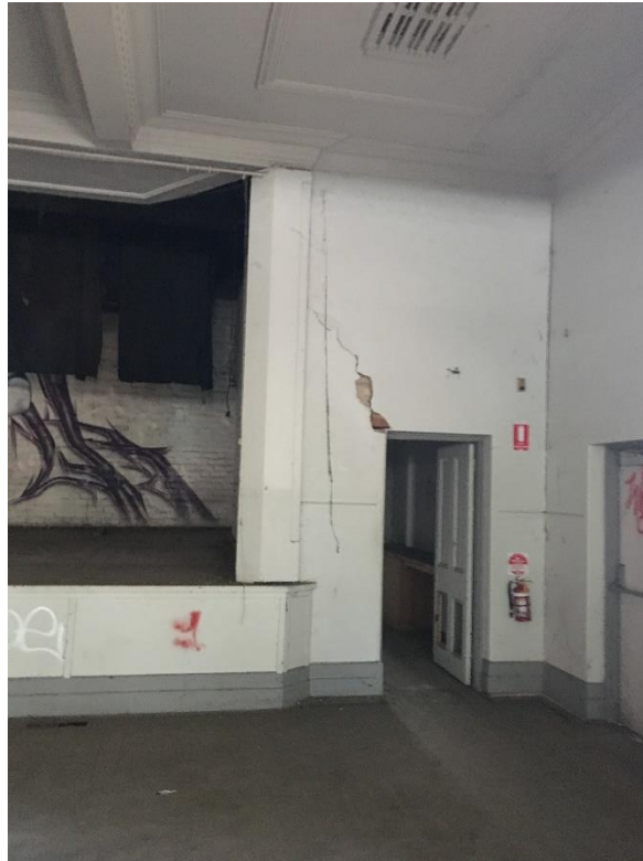
Photo 16: Cracking above door (leading from Hall (9) to Room 10A, cracking looks to not have gotten worse since previous report.
