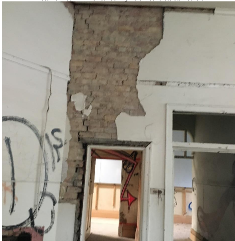
Photo 19: Large cracking at internal wall, room 1/6 interface
