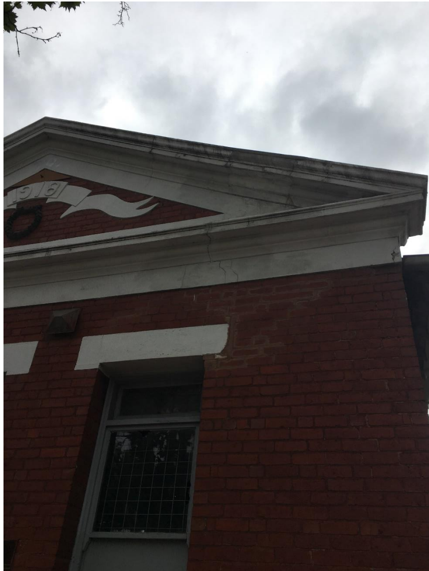
Photo 11: South-West corner of Hall – west wall. Cracks to wall repaired externally. Internal crack not repaired.
