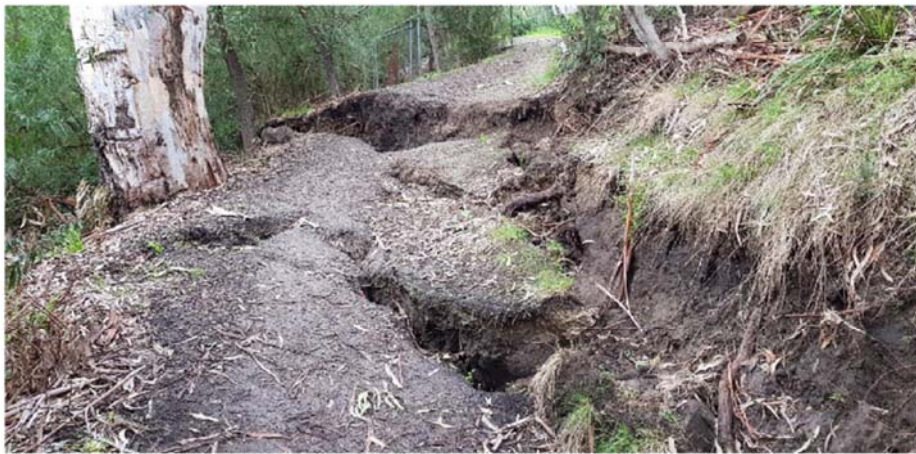
Figure 2. Tree (T1) and bank slump site visit by Alluvium
