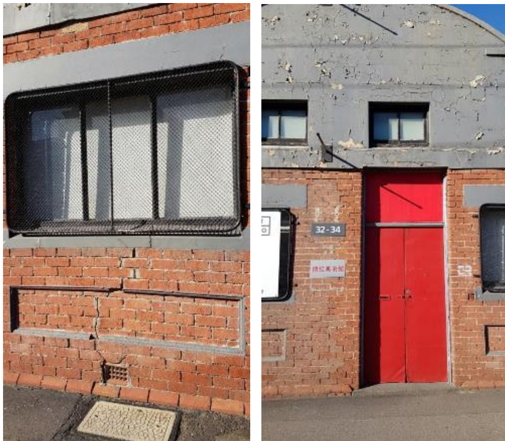
Figure 26. Details of the façade showing window and decorative panel (left) and doorway (right). Source: Trethowan Architecture 2019.
