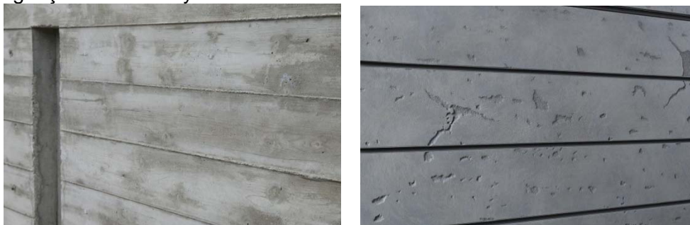
Examples of concrete walls with horizontal joint lines provided by Council's Heritage Advisor
