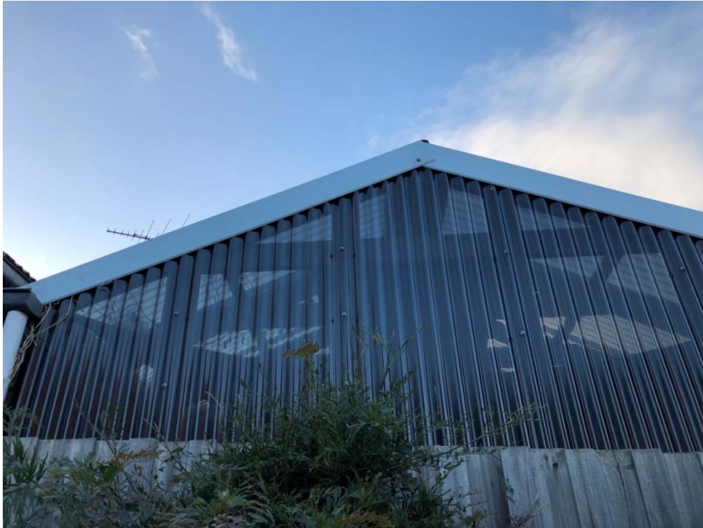
Image 7: The enclosed structure of No 10 Rogers Street, taken from No 16 Derby Street, facing east
