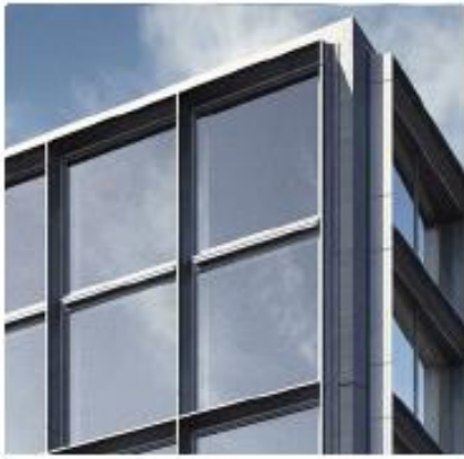
Podium - External metal framing
