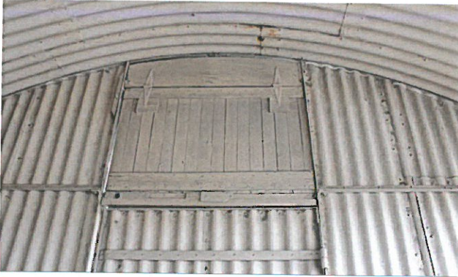
Figure 7 Detail of opening & door, east elevation. Note original timber infill above the opening.
