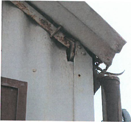
Figure 8 Detail of typical damage, west elevation.
