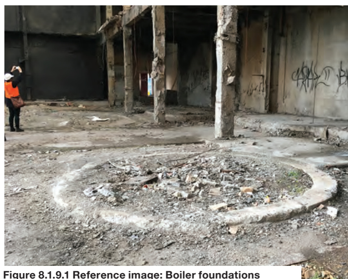
Figure 8.1.9.1 Reference image: Boiler foundations
