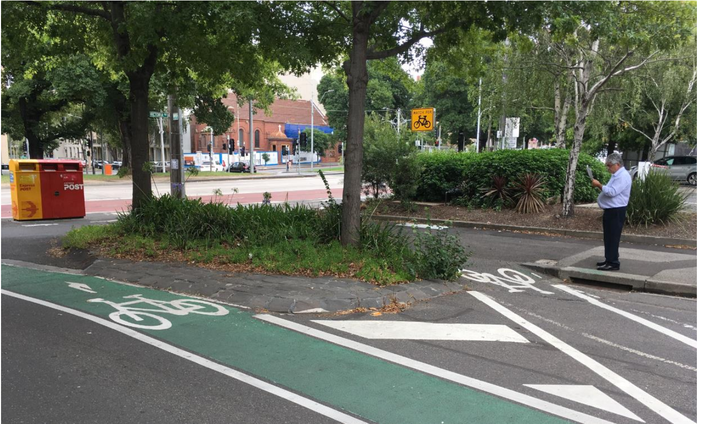
Existing extension, west side of Napier Street – to be demolished as part of the traffic improvement works.
