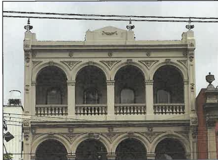
Figure 8 The truncated parapet has been partially reinstated with new urns and a central parapet, though it seems likely that these works may not have restored the parapet to its complete, original configuration. One of the urns is now missing.
