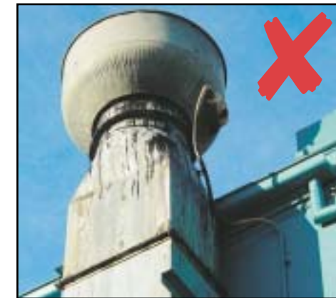
EXAMPLE OF GREASE LEAKING FROM A DIRTY EXHAUST FAN.
