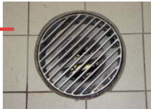
FLOORWASTE DRAIN WITH SILT TRAP AND CONNECTION TO SEWER.
