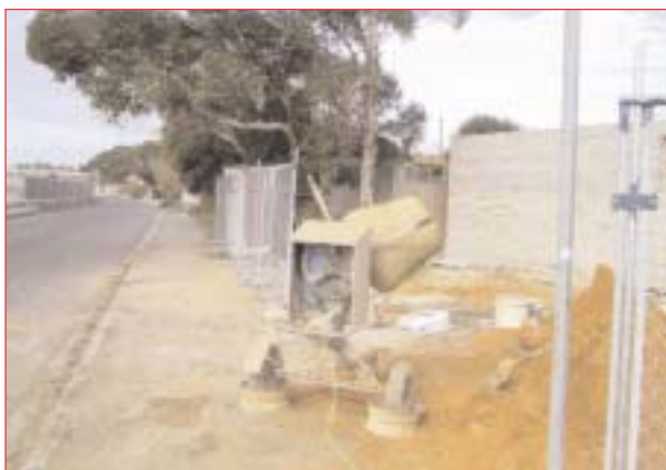
Unacceptable building site
