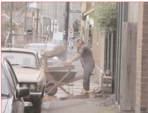
Consideration must be given to safety of workers and others who may use the footpaths.
