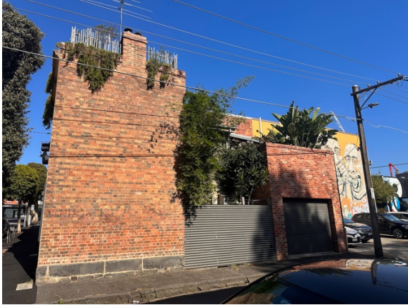
Figure 09: 8 Derby Street, frontage to Little Oxford Street, with subject site at right and behind.
