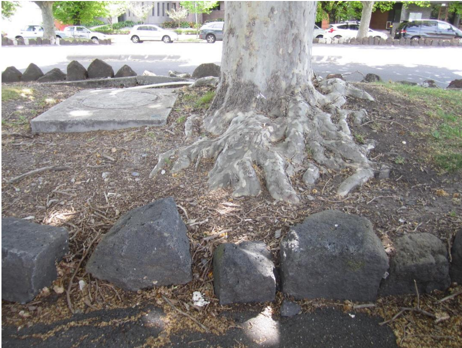
Figure 7: Damage to the median border caused by roots of the London Plane.
