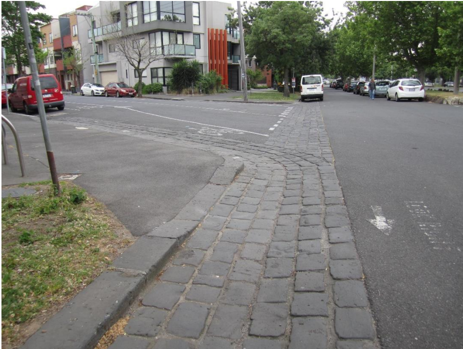
Figure 19: Northern drainage channel configuration of six rows of basalt pavers continues across the intersection of Napier Street and the Queens Parade service lane, terminating at the intersection with Jamieson Street.
