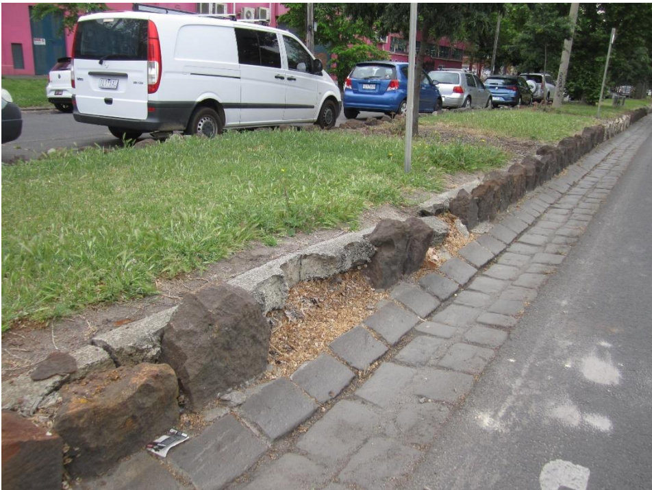
Figure 10: Median between Alexandra Parade and Napier Street. View of missing uncut basalt blocks and basalt pitcher drainage channel.
